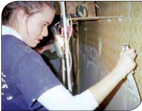
Student helps to repair house of a flood victim in Baileysville, WV.
